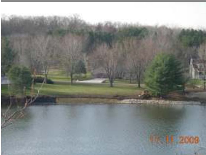
Frank & Carol Durkin and east end of the RCD's West Beach Shorelines, Stabilization IN PROGRESS...
